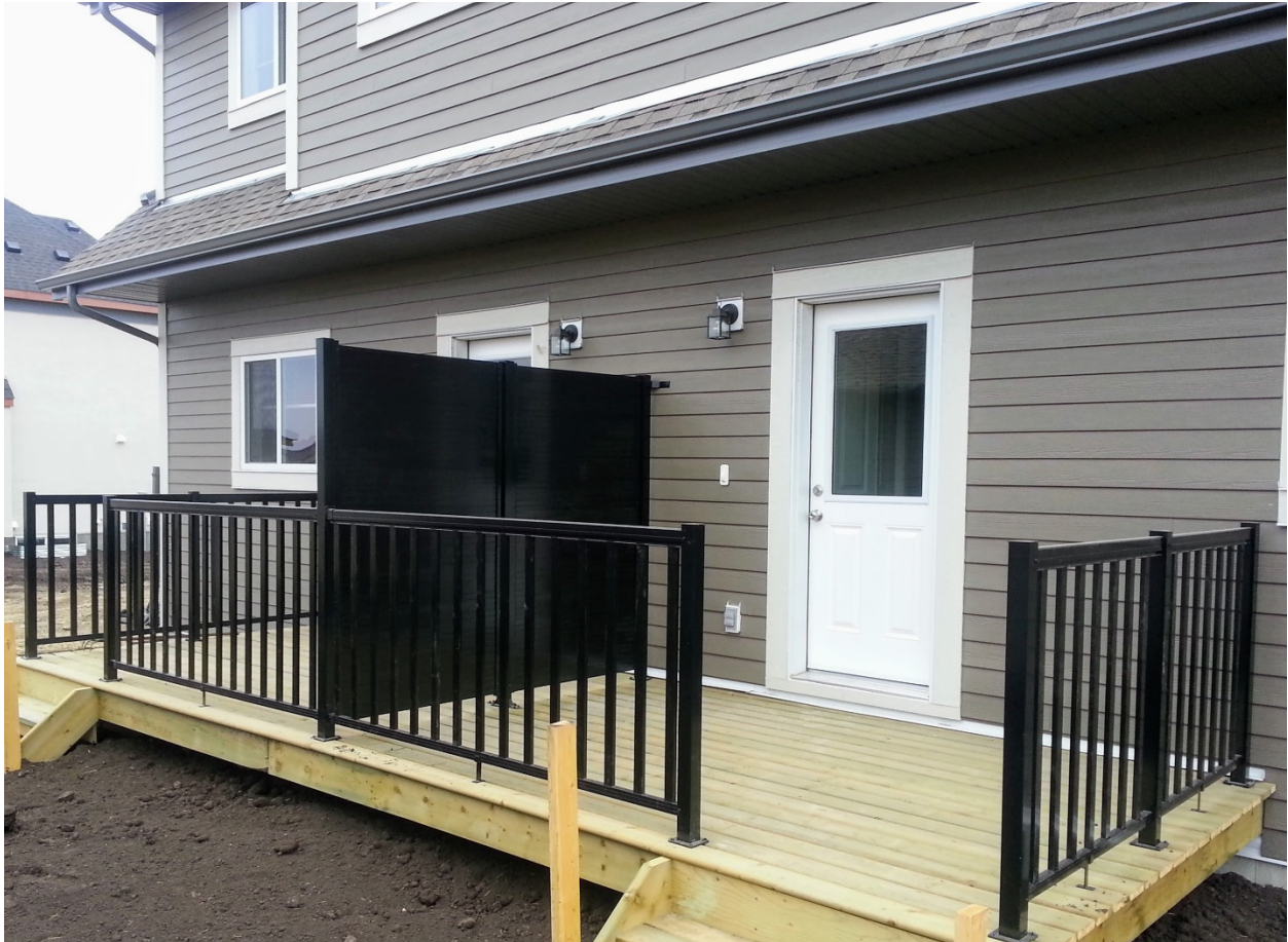
Figure 4 6-foot Wind Wall
